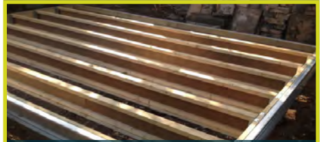
QuadraPile foundations support the modular galvanised steel & timber perimeter beams & timber floor structure.
